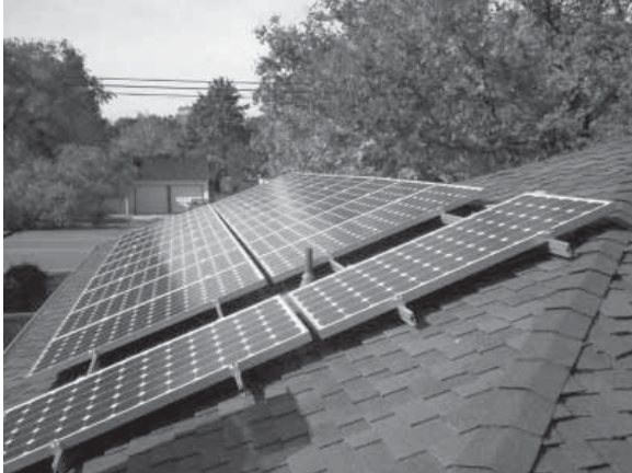
Photovoltaic roof panel
